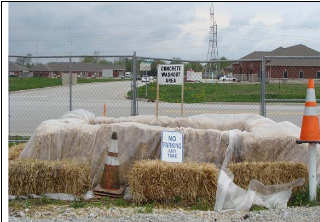
Concrete washout with plastic liner along with sign clearly marked "concrete washout area".
