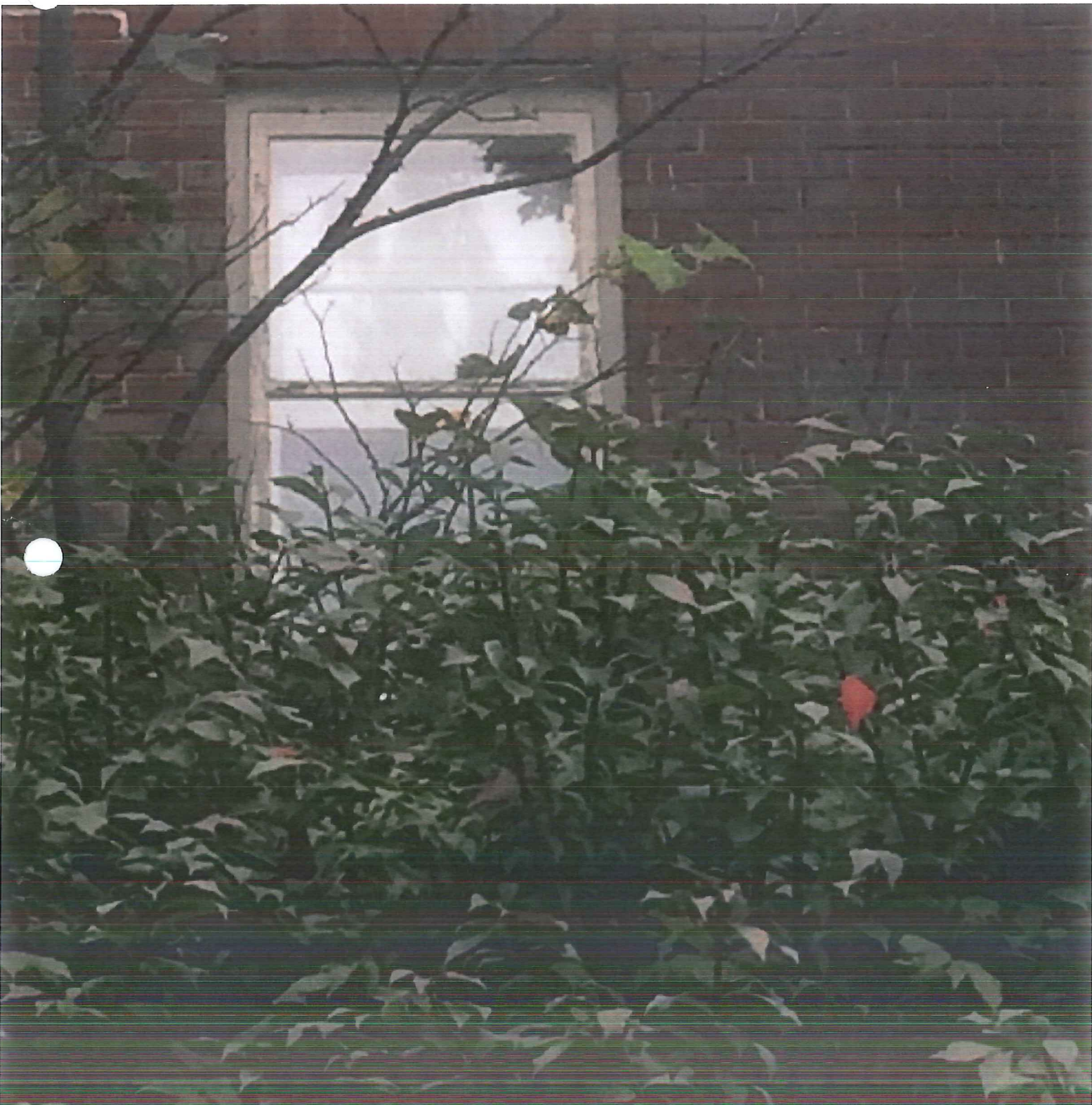
Window to be replaced
